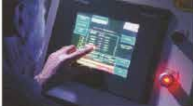
All system functions and parameters are accessed by simply touching the HMI/M4 control display.
